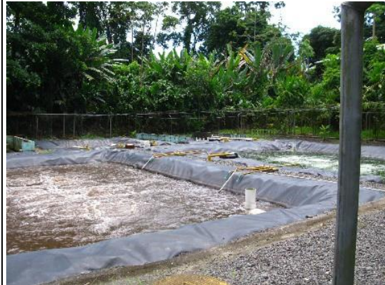
Photo 162: I-17 Wastewater treatment plant on site
