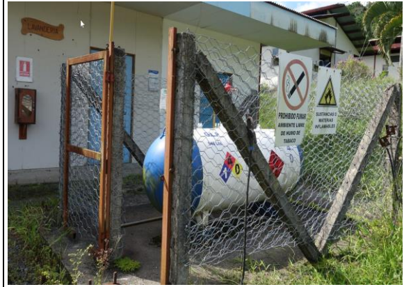
Photo 38: I-3 Fuel storage showing safety and drainage measures
