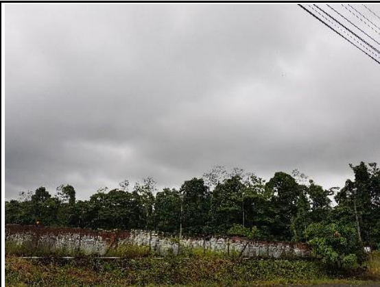
Photo 171: Old transformers from the temporary distribution lines that were used throughout the construction areas (I-18)
