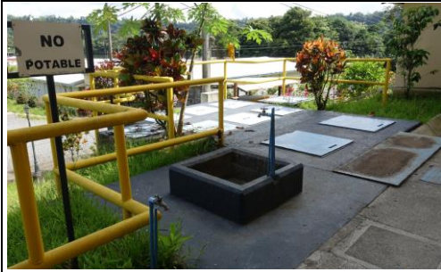
Photo 43: I-3, I-12, I-18 Water and liquid waste management in kitchen area
