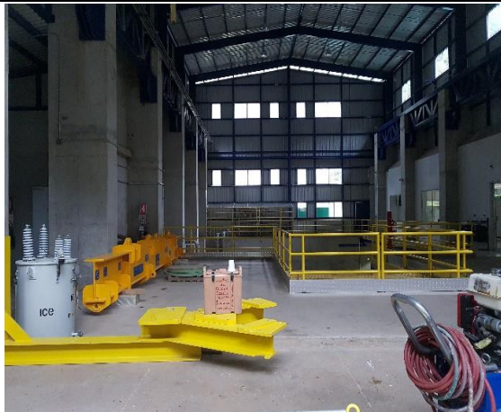
Photo 48: Inside of remotely operated ecological flow power house (I-4).
