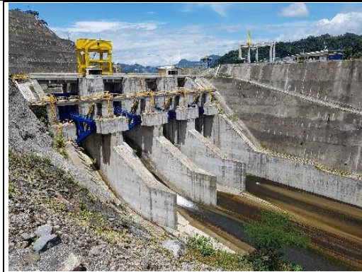
Photo 60: View of spillway with leak in left-most bay (I-5)
