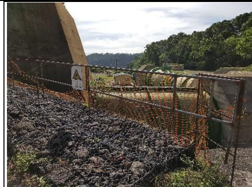
Photo 55: Protective fencing in need of repair at the surge chamber (I-5)
