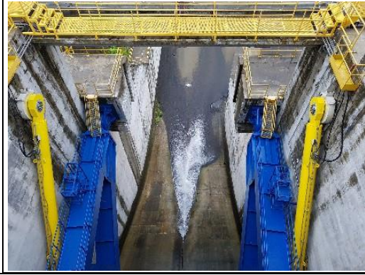
Photo 63: View of leak between concrete blocks in left-most bay of spillway (I-5)
