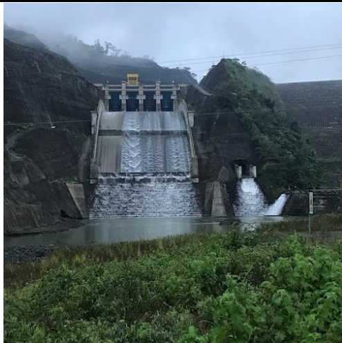
Photo 181: I-20 View of the spillway from downstream, with bottom outlet to the right
