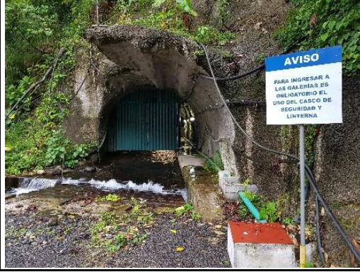
Photo 68: Dam gallery and seepage flows near right side of the dam adjacent to spillway (I-5)
