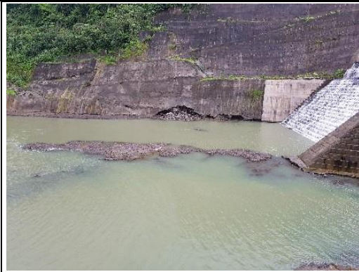
Photo 66: Downstream from spillway, right bank erosion (I-5)
