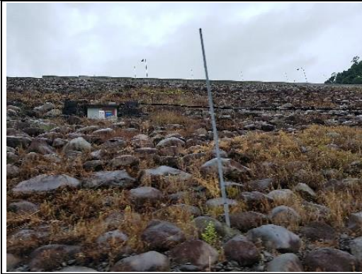
Photo 64: Downstream face of dam with instrumentation hoses and weeds treated with pesticides (I-5)
