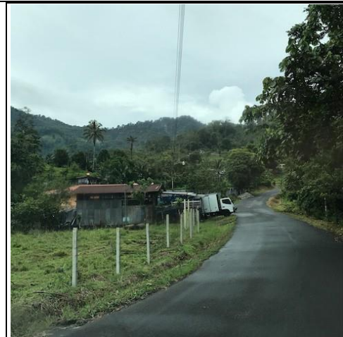
Photo 76: I-7 Part of the re-surfaced road, Ruta 415, from El Cruce to Bonilla on the left bank
