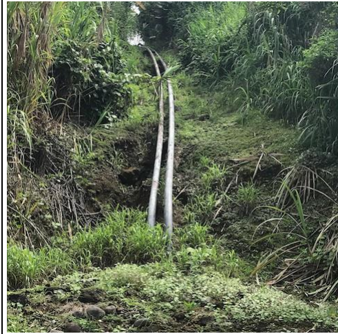
Photo 101: I-9 Gas pipeline section near Santa Marta; the line runs from Limón to San Jose and passes close to PHR
