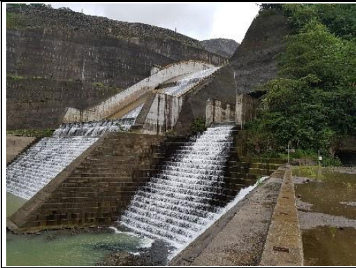
Photo 67: Energy dissipators downstream of spillway and low level outlet. Seepage flow from dam galleries is discharged towards the right hand of photo (I-5)
