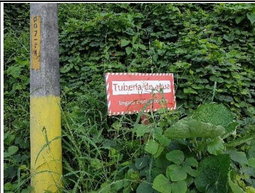
Photo 54: Water pipeline for fire at the construction camp. (I-5)
