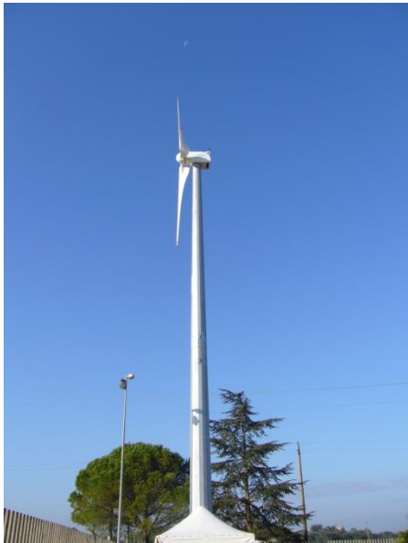
G- Turbina eólica 20 kW full-converter
